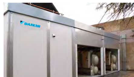
MCP with Dual Chillers Inside
